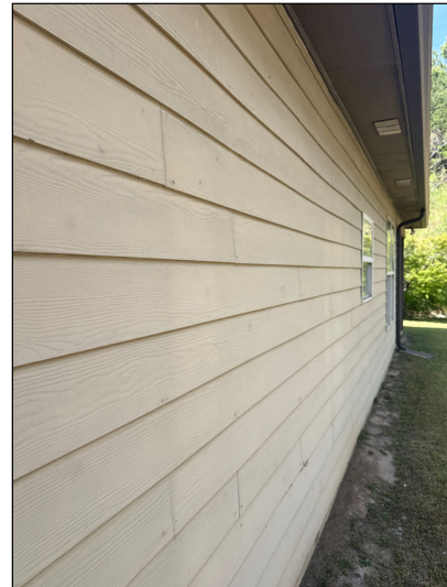
Caulking/Sealant of butt joints, gaps, cracks and have started to fail.
