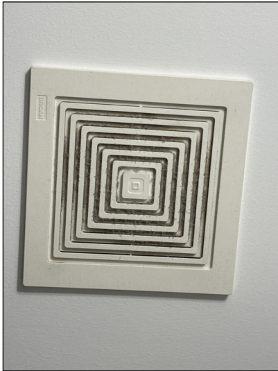
Dirty fan, preventing properly airflow.
