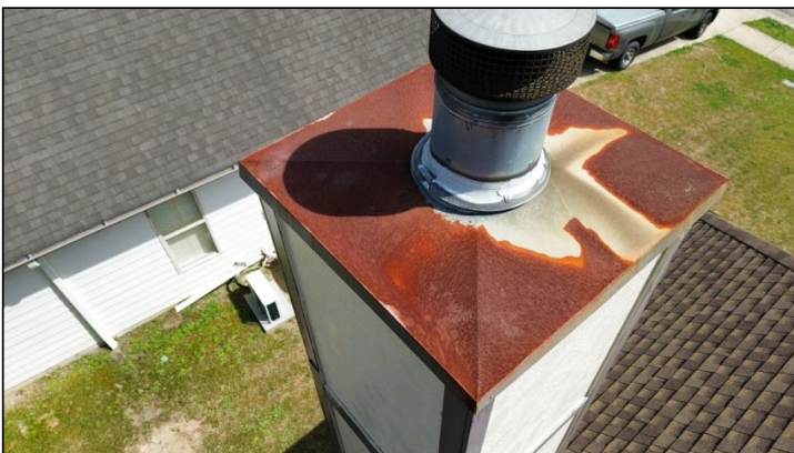
Rusting observed on chimney cap.
