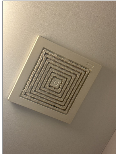
Dirty fan, preventing proper airflow.
