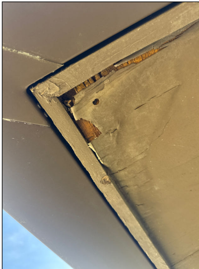
Wood rot observed on soffit corners. Recommend review for repair as necessary.
