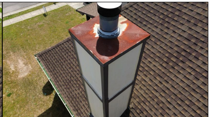
Rusting observed on chimney cap.
