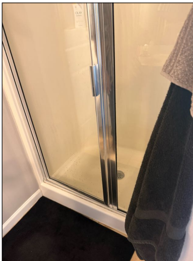
Shower door doesn't close properly. (Gets stuck at bottom corner.)
