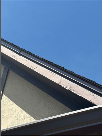
Peeling paint observed, suggest scraping and painting as necessary.
