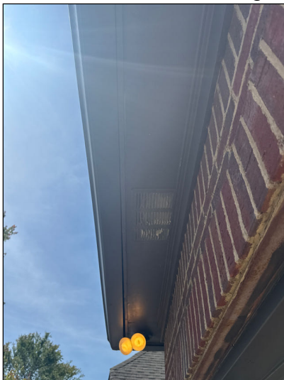
Soffit vent needs cleaning, to help provide adequate attic ventilation.
