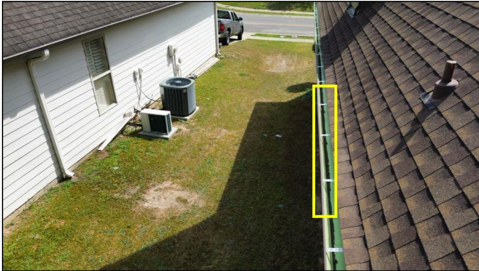
Small amounts of granules from shingles noted.
