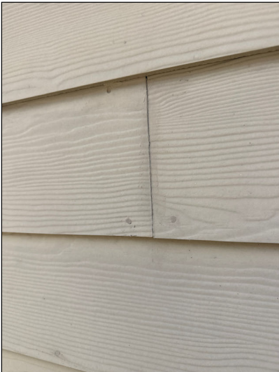
Caulking/Sealant of butt joints, gaps, cracks and have started to fail.
