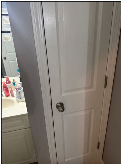
Doesn't latch properly
