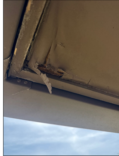
Wood rot observed on soffit corners. Recommend review for repair as necessary.
