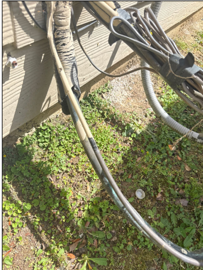
Missing/damaged insulation at A/C unit.
